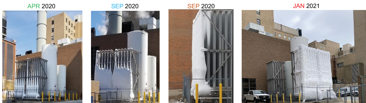
Fig. 1. Increased demand for liquid oxygen resulted in progressive icing of the heat exchange coils.
