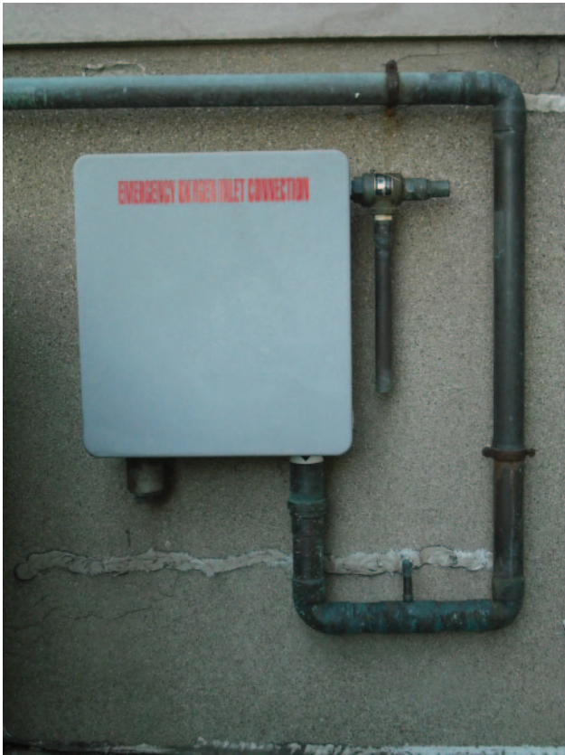
Fig. 3. University Hospital emergency oxygen inlet.
