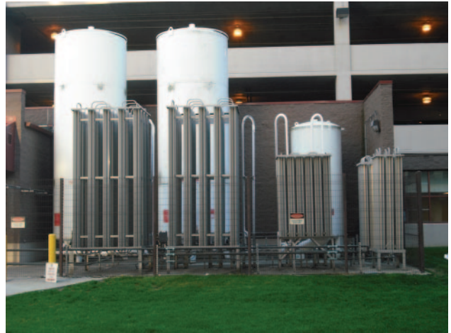
Fig. 2. University Hospital liquid oxygen system.
